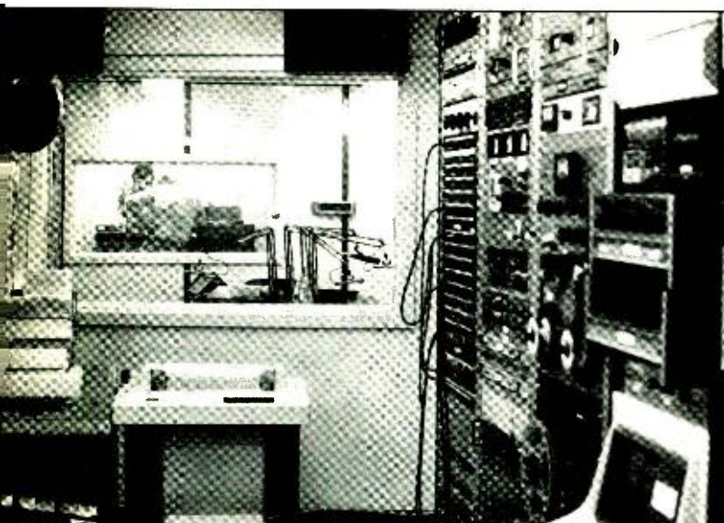
View from main control room looking into the on-air interview and newsroom, with mic stands around table. Beyond that is production control room
