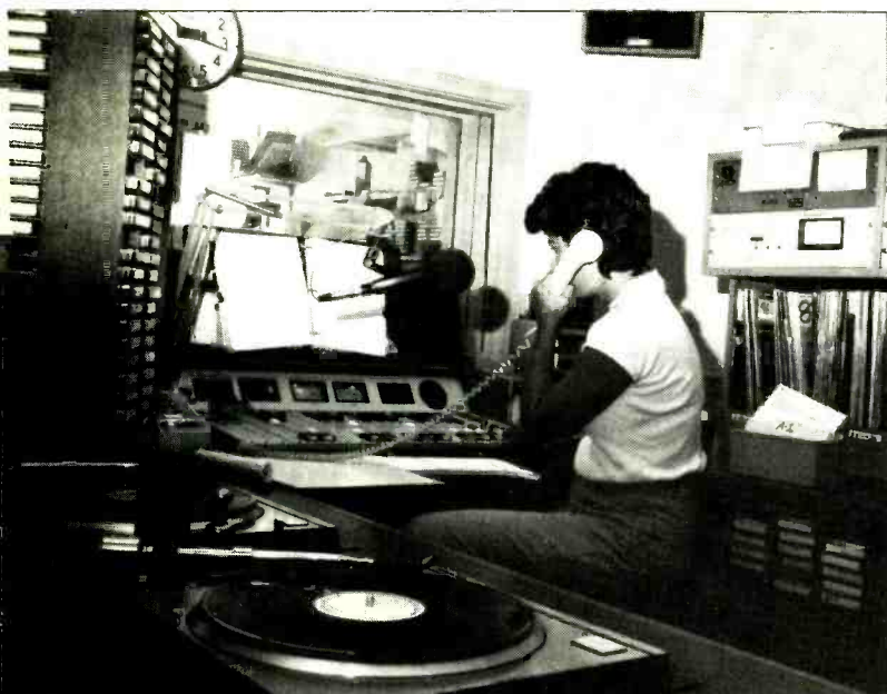
AM studio is between production room and news studio, and is, like other rooms in plant, laid out for high efficiency in a small space. Discs are in racks at right, carts at left
